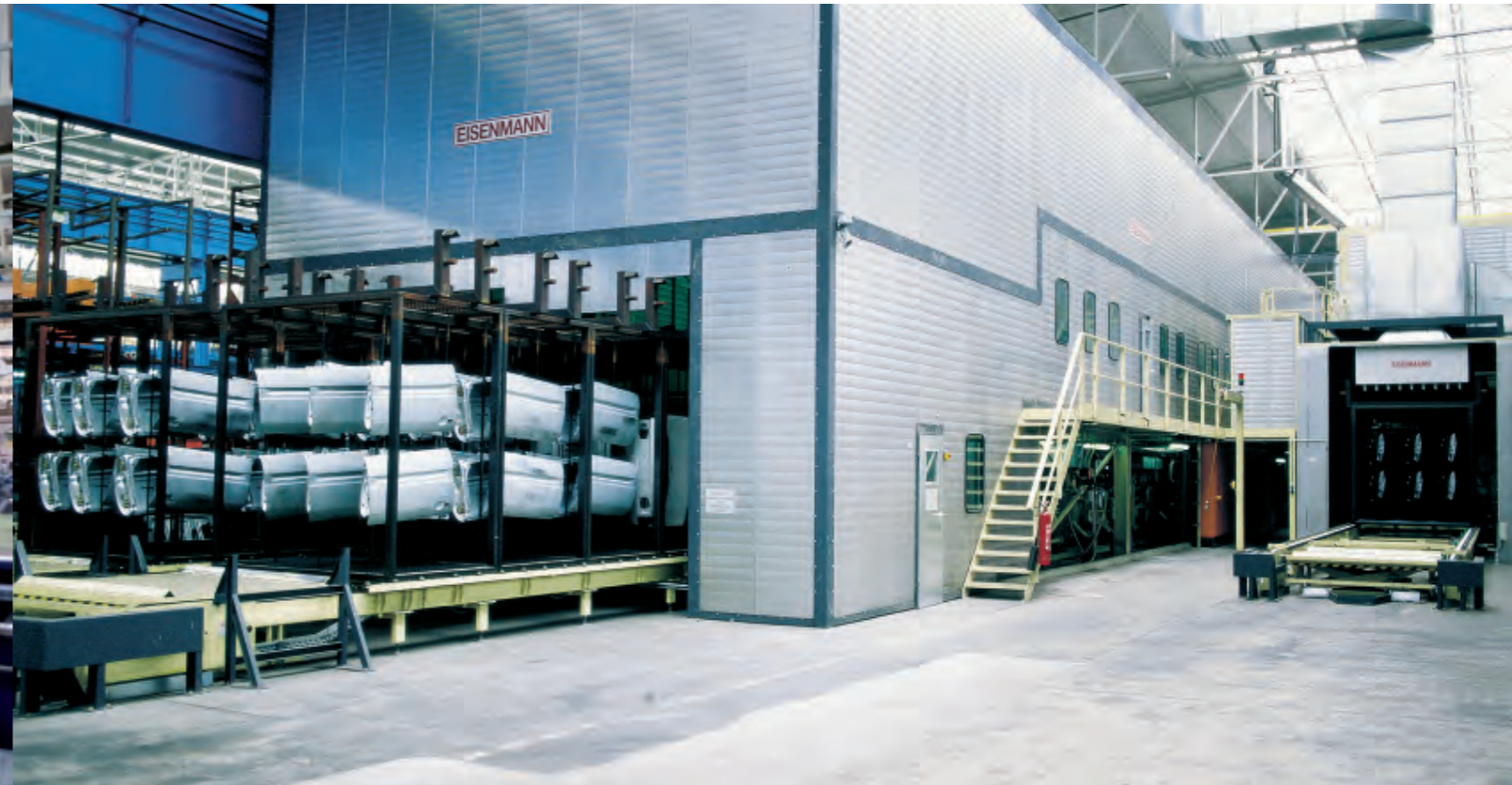
Cathodic top coat curing oven with bottom entry/exit for heat loss prevention.
