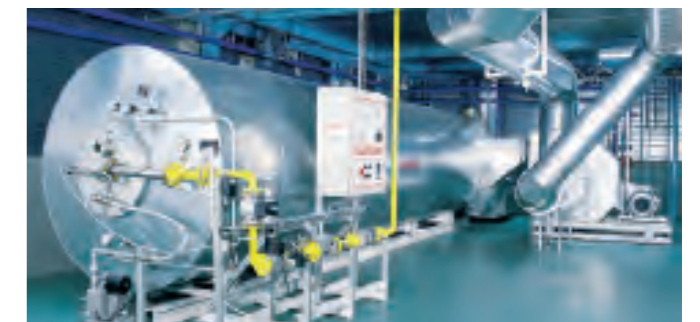
Thermal oxidizer with heat recovery for purifying exhaust air from the E-coat curing oven.
