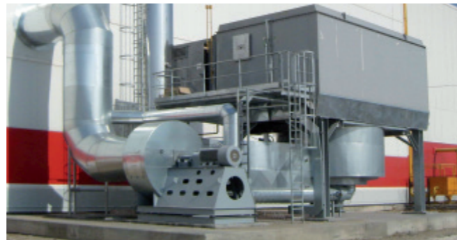
Regenerative thermal oxidation (RTO) with rotating distributor to minimize pressure fluctuations.
