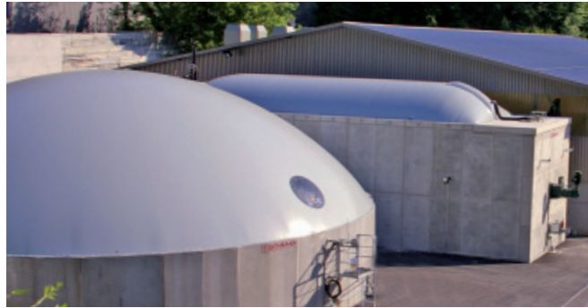
Digestate storage tank and horizontal plug-flow digester made of pre-fabricated concrete elements.
