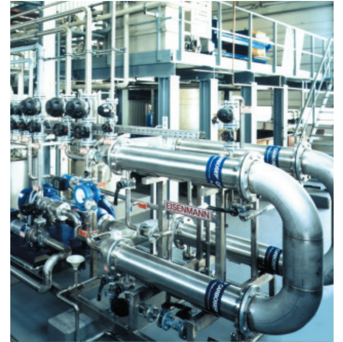
Ultrafiltration with tubular modules for emulsion splitting at a waste-management facility.
