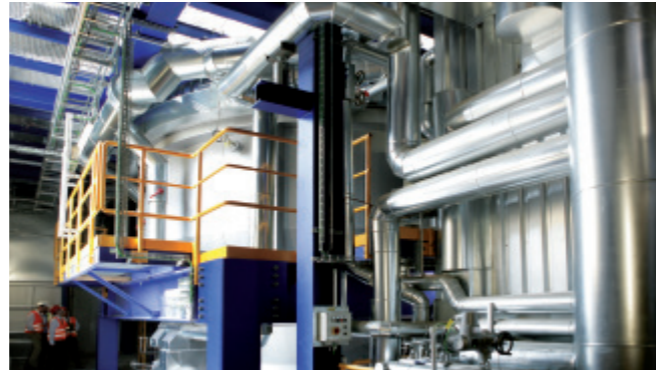
Fluidized bed incinerator for processing oil shale at a cement plant.
