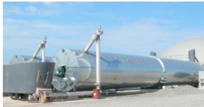
Horizontal digester made of steel.
