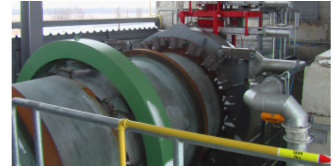
The rotary kiln with a refractory lining ensures safe, long-term operation at temperatures up to 1,200°C. It is used for the disposal of rocket propellant.
