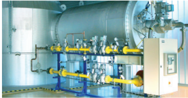
In the Turaktor® – a high-turbulence combustion chamber – gaseous and liquid by-products of detoxification/neutralization processes are incinerated at 1,200°C.
