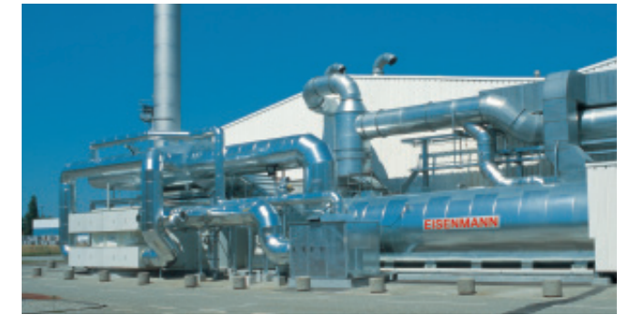
Exhaust air purification with an adsorption wheel and TO in the chemical industry.
