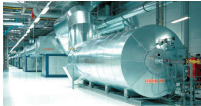
Exhaust air purification with thermal oxidation (TO).
